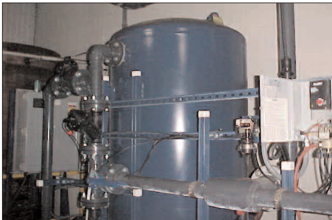
Above: Multimedia filter. Right: Duplex water softener.
